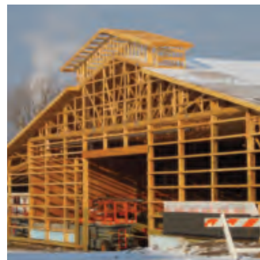
Construction has been coming along nicely on the 27,000 square foot arena, which replaces the old Judging Arena at the Minnesota State Fairgrounds.
